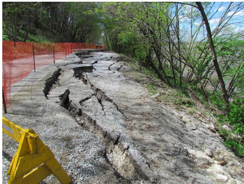
Figure 10 Deteriorating route conditions along Great River Road in Lee County
